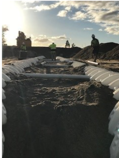
Picture showing balancing pipes
