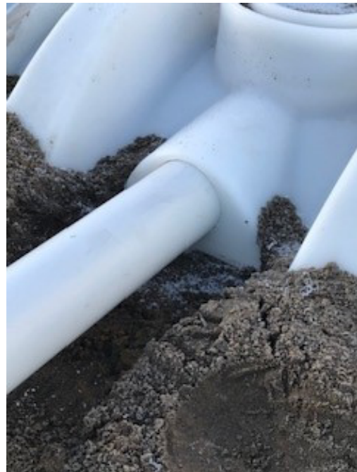
Un-sealed awaiting mastic
