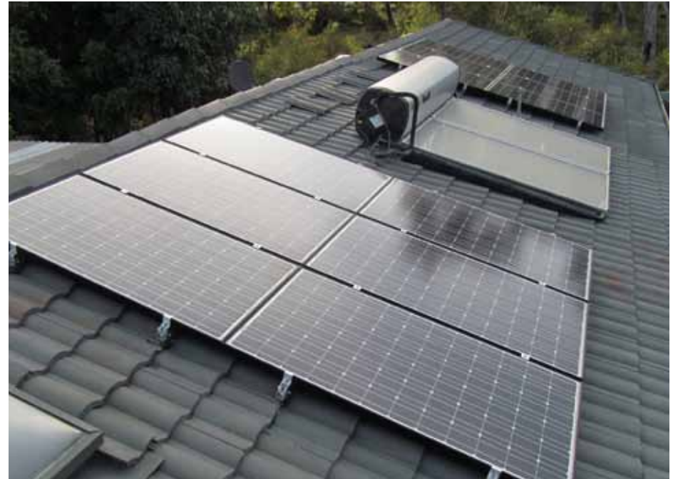
Solar panels and a solar hot water system help to reduce power costs
