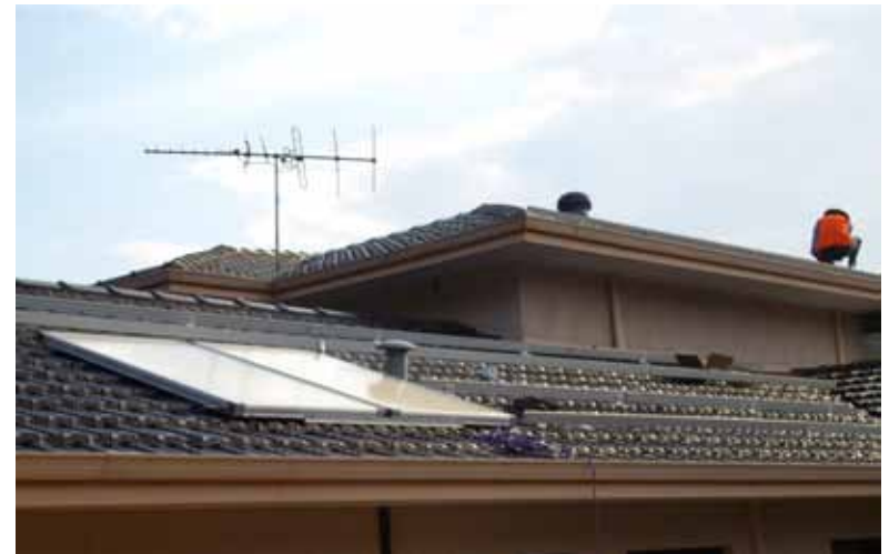
Installing solar panels can help to offset carbon pollution
