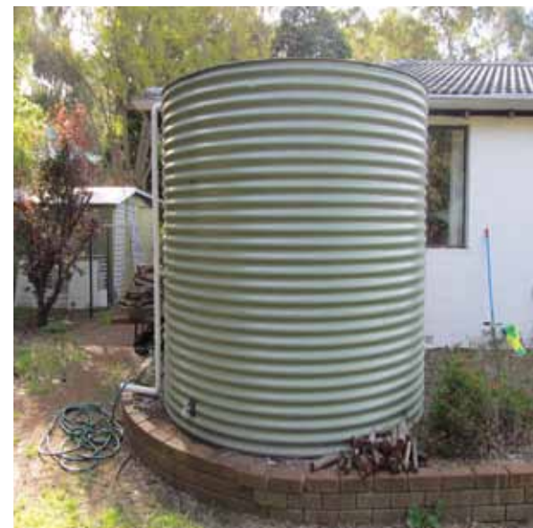
A tank installed in a home in Gooseberry Hill
