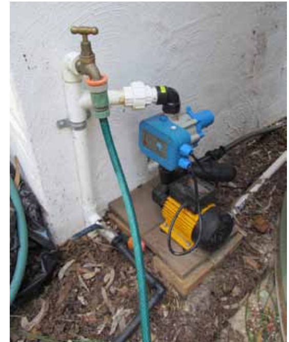
Electric pump on a water tank, capable of opening and closing the valve Photo courtesy of Steve Gates
